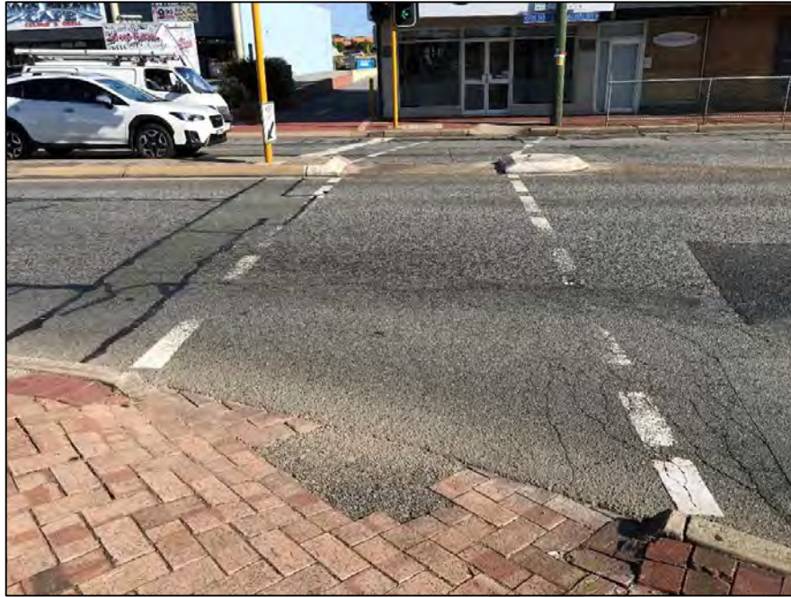
Finding 2.8 – Poor ramp maintenance and not correctly aligned.
