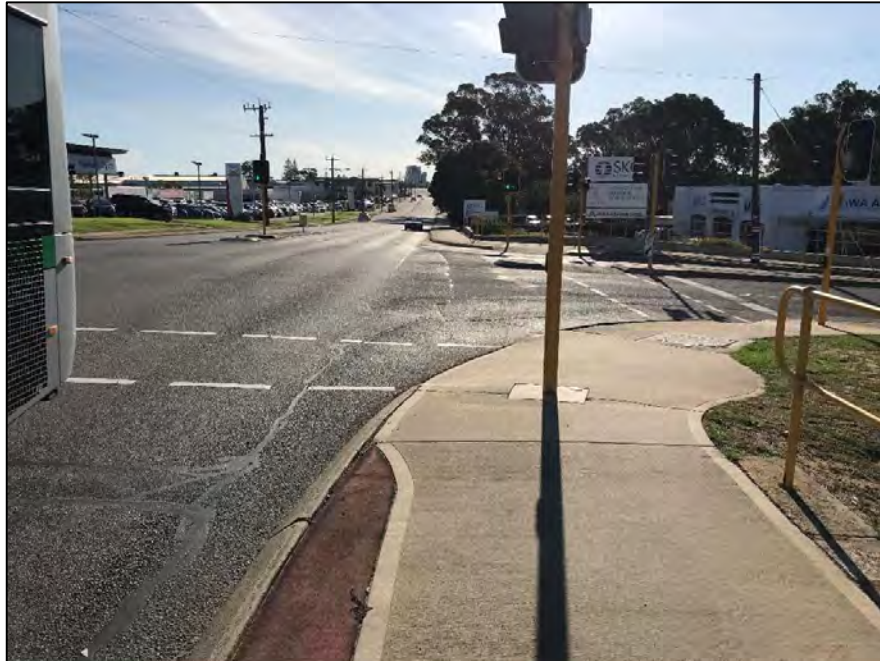
Finding 2.10 – Path Obstructions - traffic control signal post located in path.
