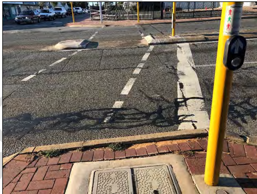
Finding 2.8 – Poorly aligned pedestrian crossing. Ramp not in line with line marking and too narrow.
