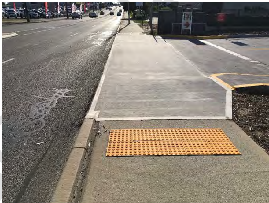
Finding 2.8 – Inconsistency with the installation of TGSI - the above location is at the entrance to a service station.
